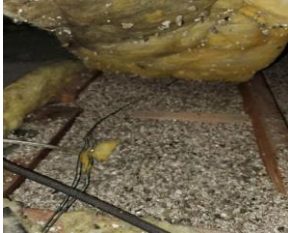
Vermiculite attic insulation
