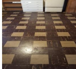
9"X9" asbestos floor tile
