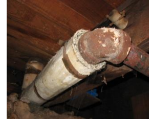
Asbestos pipe insulation
